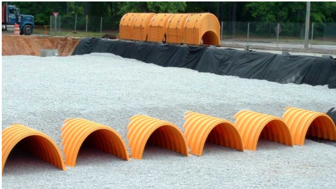
Fig.14 - StormTech Attenuation System
